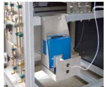
Acid pump for nitric acid
