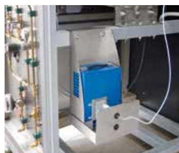
Acid pump for nitric acid
