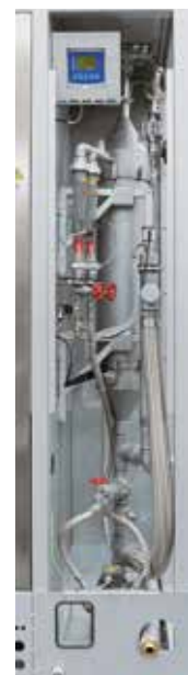
Scrubber to clean generated process gases by washing out
