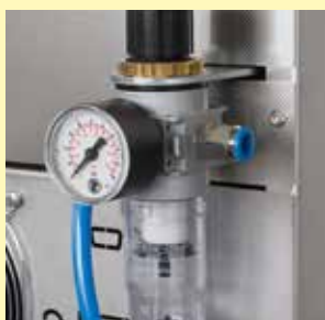
Forced cooling system with compressed air
