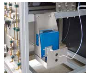
Acid pump for nitric acid
